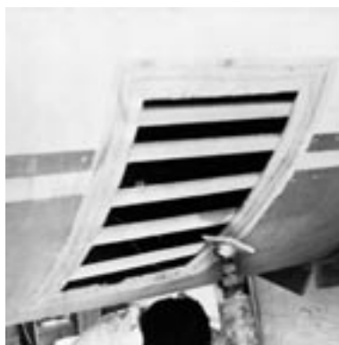
Figure 6-16 Bevel the edges and fasten temporary stringers to the back of the opening.
