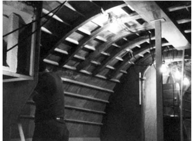
Figure 26-4 Interior construction in an upside-down hull of an IOR ½ ton racer. Lighting and tools are set up in the hull. Note the band saw in the background at the far right.
