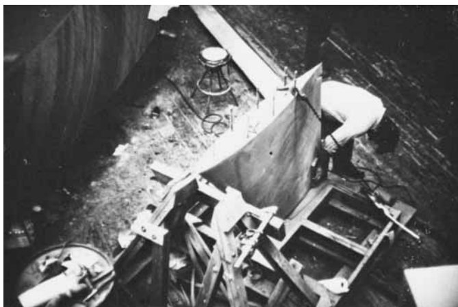
Figure 14-23 A keel set up in a specially-built handling fixture so it can be final faired and moved around.
