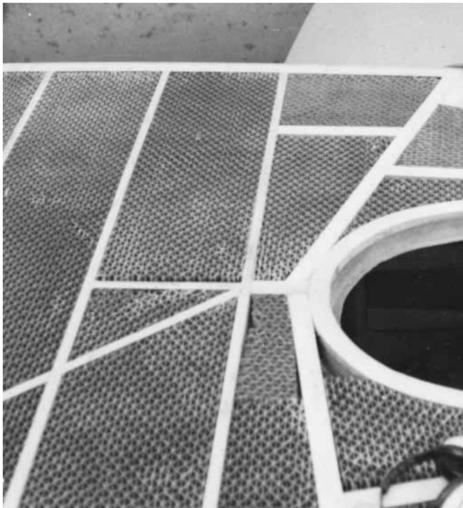
Figure 11-14 A cored deck constructed using lightweight beams and resin-coated paper honeycomb core material. See Chapter 27 for a full description of this deck construction.
