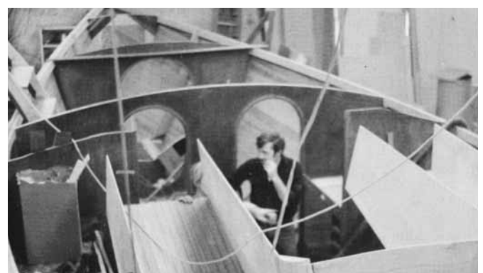
Figure 27-13 An unusual slingshot-shaped cockpit is set in place on Golden Dazy . It is trued up with temporary bracing and blocking. Then the deck framework is installed around its perimeter.
