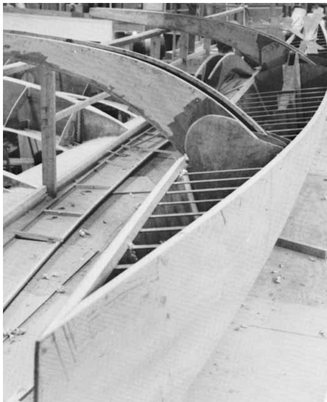
Figure 25-26 Tension flanges for deck I-beams are bonded to the underside of the sheer clamp. Sheer webs for deck I-beams will be bonded to the top of these flanges. They will look like the deck beams in Figure 25-24.
