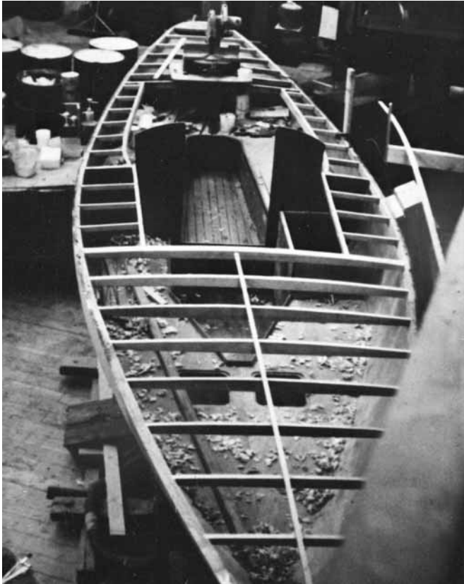
Figure 27-31 The deck of a 26' (7.9m) Luders 16 framed-in and ready for plywood covering.
