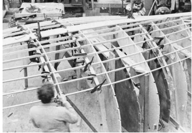
Figure 22-11 Laminating floors over stringers. To ease the job of laminating and installing floor timbers, it was done before the topside stringers were installed.
