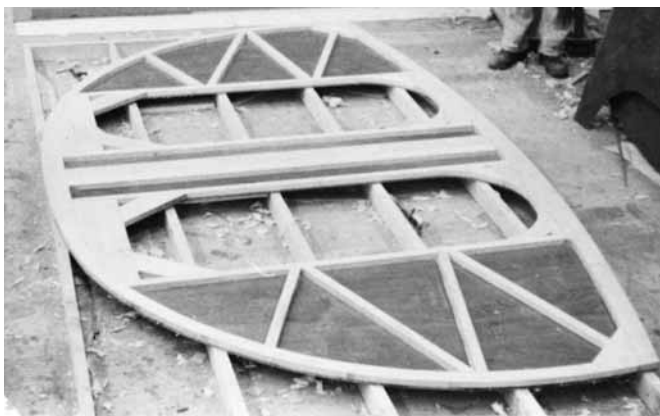
Figure 26-12 A major structural bulkhead for Golden Dazy is constructed with a framework sandwiched between two \frac{1}{2} " (12mm) thick panels of utility plywood.
