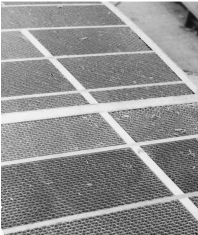
Figure 27-25 A sandwich deck with all of the framing and honeycomb core in place before the top plywood deck surface was laid.
