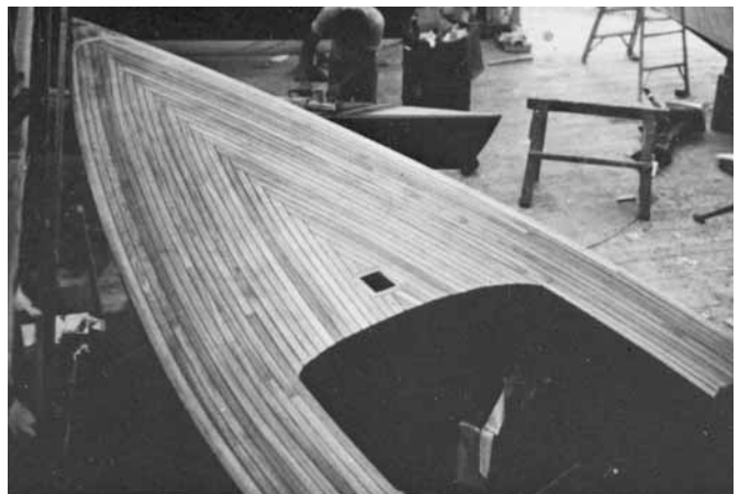
Figure 27-34 Deck planking and final sanding are completed. Note the herringbone pattern where planks meet along the centerline. Also note that the teak begins several inches inboard from the sheer to allow for a painted cover board for an attractive effect.
