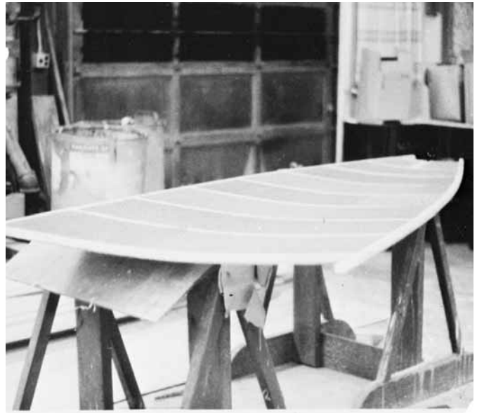
Figure 11-16 A cockpit sole with a curved shape using core laminates. This was accomplished by laminating a curve in the frames before they were bonded together.
