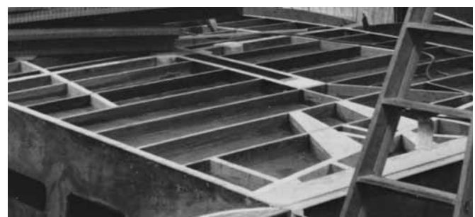
Figure 27-23 Sawn Sitka spruce blocking is bonded to core deck at all structural frames and planed flush with the deck profile. Note the strip of blocking for adjustable sail leads to the left.
