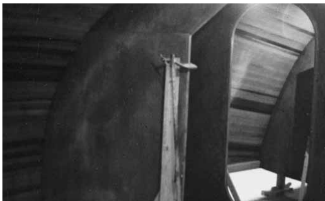
Figure 23-10 The 42' hull with the temporary mold removed. The hull is supported by permanent bulkheads installed during set-up. Note the clean interior in which work can progress while exterior finishing is completed.
