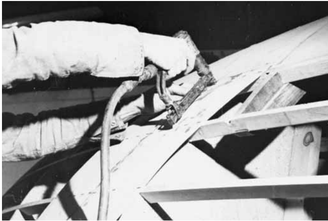
Figure 22-14 Stapling the first layer of planking to the topsides. Note the laminated curved frame and blocking in the upper right as well as limber holes cut in stringers next to blocking.
