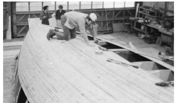
Figure 23-4 Strip planking a 42' (12.8m) hull. These strips are being laid from a master plank from the bilge up to the keel.
