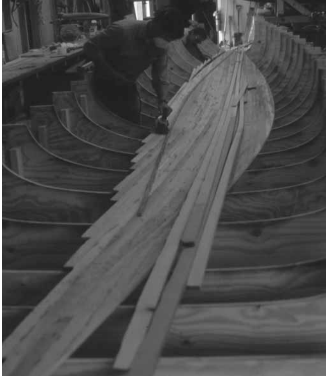
Figure 23-14 Planking being installed on a mold for the hull of the Formula 40 trimaran Adrenalin . The hull was built in left and right female molds rather than the typical male hull and deck molds.
