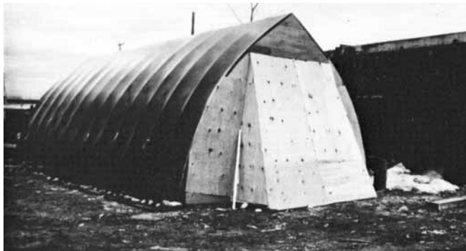
Figure 8-18 Shelter completed. Plywood walls were used at both ends to give the structure extra rigidity.
