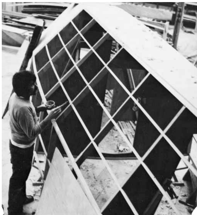
Figure 24-8 Applying adhesive mixture before bonding a panel to the framework. The panel lying against the framework in the foreground will be scarfed in place.
