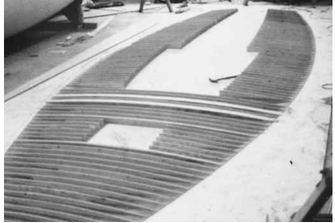
Figure 27-21 Scrap strips of plywood are used as core framing for a sandwich deck.
