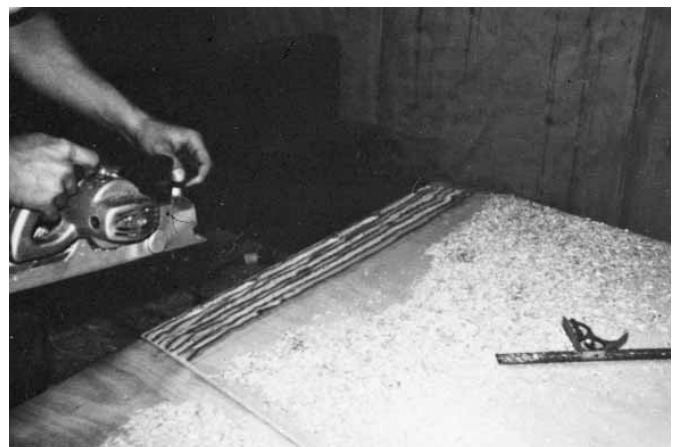
Figure 12-10 Use a power plane to rough shape a scarf bevel. Finish shaping the bevel with a block plane.
