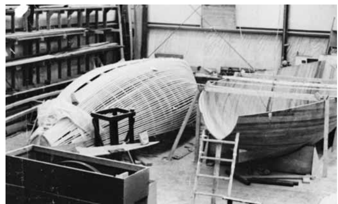
Figure 21-25 The hull is in a cradle and immediately trued up with the waterlines. Temporary bracing at the sheer stabilizes the shape of the hull while interior joinery is installed. The ladder at the open transom provides easy access to the interior of the hull.
