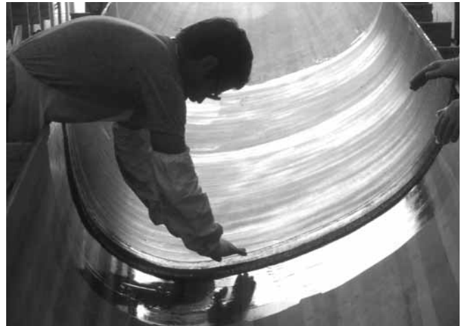
Figure 23-16 Applying unidirectional carbon fiber to the inside of the right half of Adrenalin's hull. The two halves were joined after the interior was finished and a bulkhead was installed.
