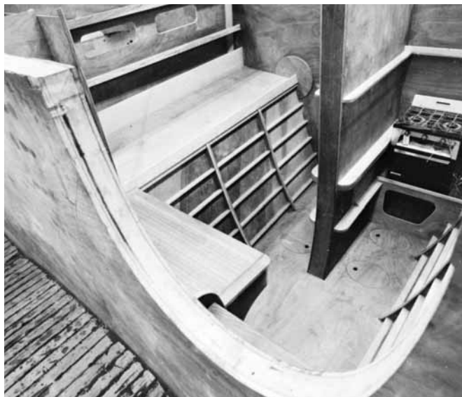
Figure 26-7 Rogue Wave's galley, pilot berth, navigation area, and daggerboard case. All interior joinery was installed before the deck was built. Circular pads on the bulkhead are reinforcing gussets. Note the lift-out access ports in the cabin sole. The unfinished teak cockpit sole is visible at the lower left.
