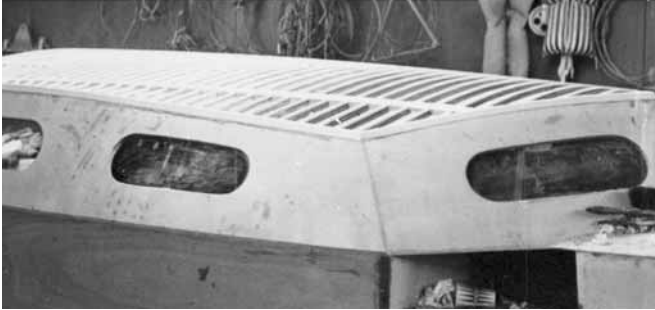
Figure 27-26 A cabin roof built over a cabin top and temporary forms inside the cabin. Small, \frac{1}{2} " wide \times \frac{3}{4} " thick (12mm \times 18mm) ribs spaced on 4" (100mm) centers were laminated over the interior ply and faired smooth. Blocking for a headsail track was inserted at the edge of the cabin and a \frac{3}{16} " (5mm) plywood roof was laminated over the assembly.
