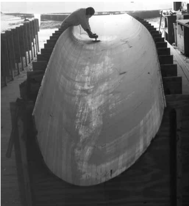
Figure 23-15 Fairing the inside of the right half of Adrenalin's hull after the cedar planking is installed.
