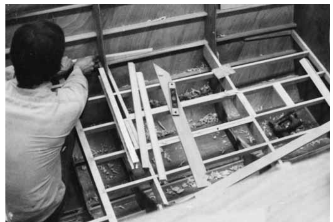
Figure 26-18 Installing cabin sole framework in Rogue Wave . The structure supports the hull skin as well as the cabin sole.
