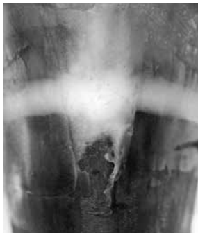
The front of a keel repair in progress. The crack has been cleaned, widened and filled with G/flex 655.
